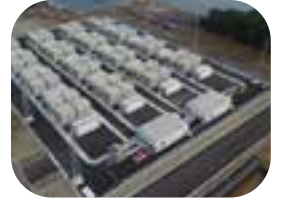
Battery storage stations
