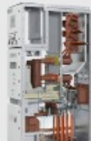
MV Panel Switchgear
