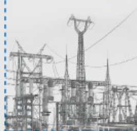
Air Insulated Switchgear
