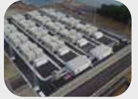
Battery storage stations
