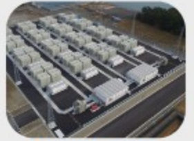
Battery storage stations
