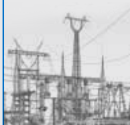
Air Insulated Switchgear
