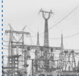
Air Insulated Switchgear
